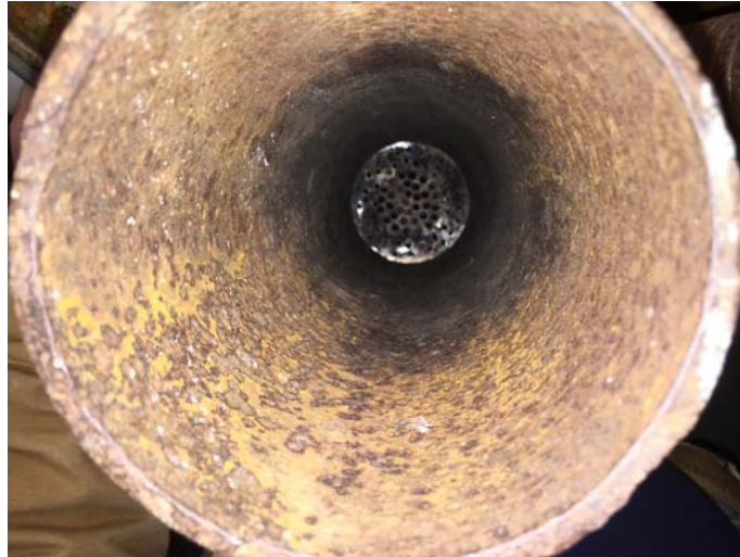
Figure 2: Four inch diameter fire tube with grate.
