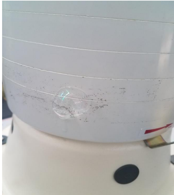
Figure 6: Main housing showing air leakage
