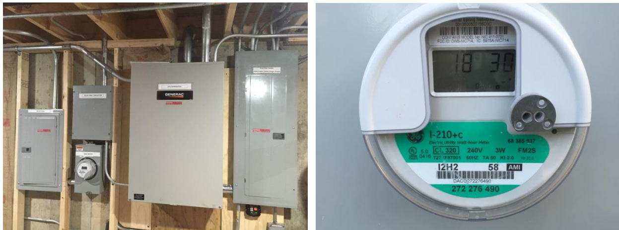
Figure 7 (a) Power Connection with SREC Meter (b) Bidirectional House Electric Meter
